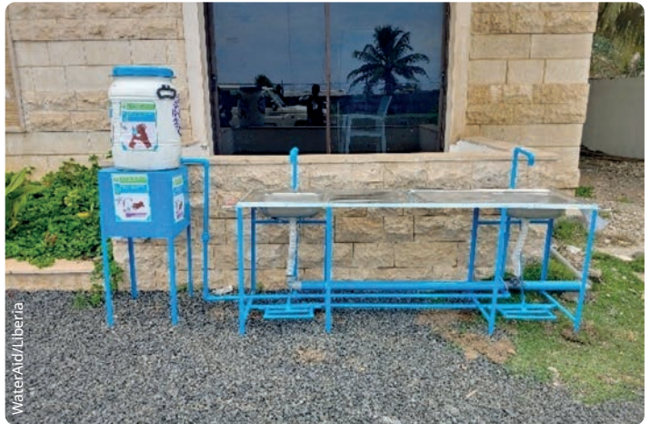
▲ ▼ Double basin handwashing facility with foot paddle.
