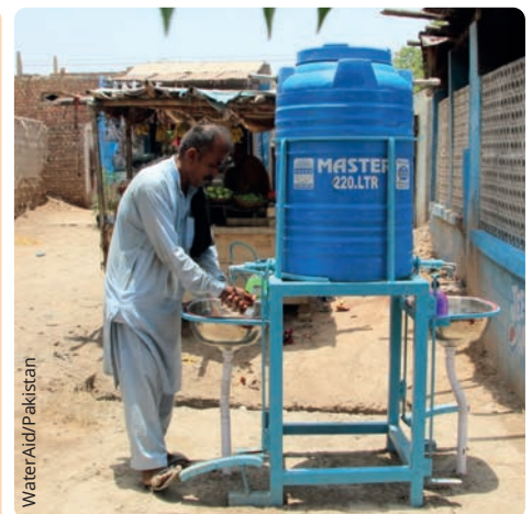
▲ A man washes his hands in Hyderabad, Sindh (Pakistan), after the installation of new hands-free handwashing facilities.
