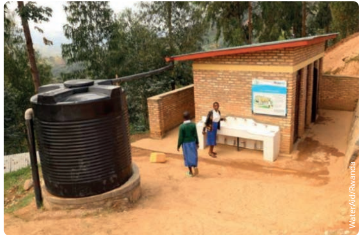
▲ Rainwater harvesting is being used for a handwashing facility for a school in Rusekera.
